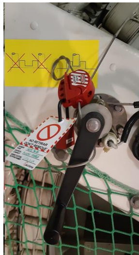
Manivela bloqueada mediante trabado de sirga y candado LOTO. Hand crank locked by means of cable device and LOTO padlock.
